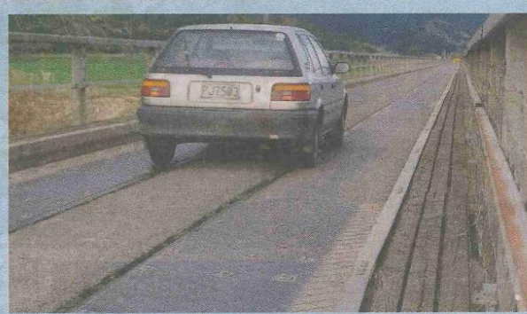
UPGRADE: The Pekatahi Bridge will be re-decked and its railway lines removed in a $5 million upgrade planned for next summer.
